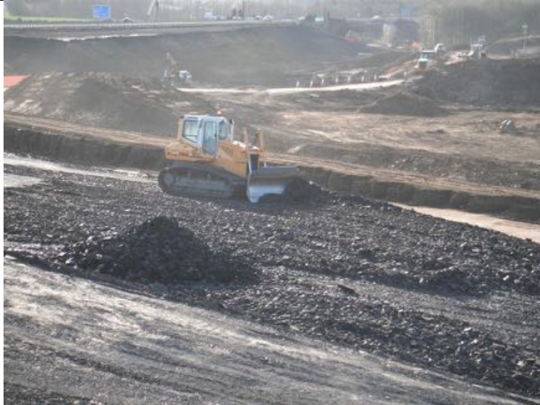
Site won granular material being graded on the Eastbound merge to the M90 Link
