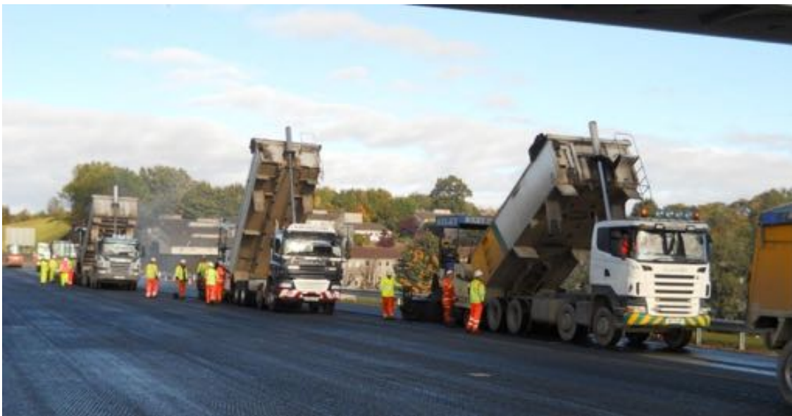
Use of new Transport Scotland TS2010 road surface specification, required echelon paving
