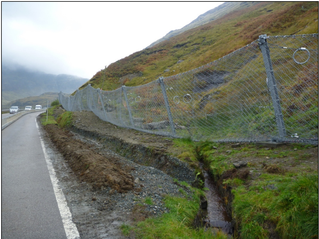
Figure 6-1: Phase 2 debris-flow barriers installed on the A83 at Rest and Be Thankful
