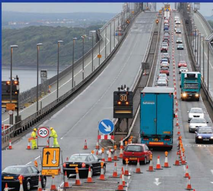
FETA's traffic management team sets out a contraflow in preparation for resurfacing of the northbound carriageway. Photo by Tony Marsh Photography, courtesy of Forth Estuary Transport Authority.
