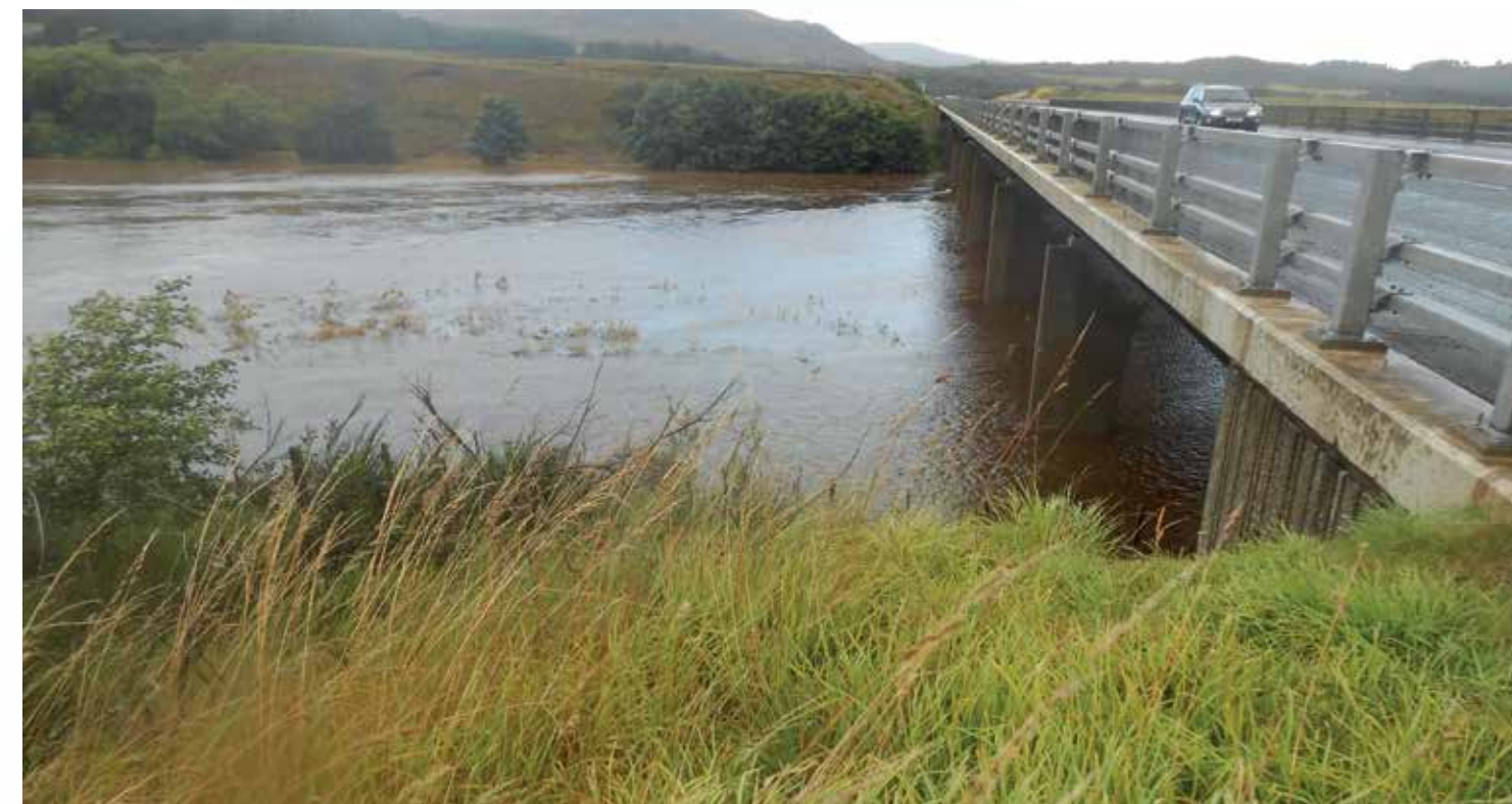
View of flooding at River Spey, looking north, August 2014
