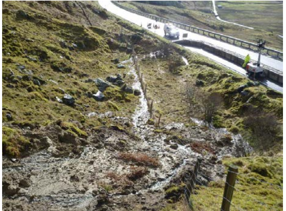
Right Landslip at A83 Rest and Be Thankful (© Crown copyright)
