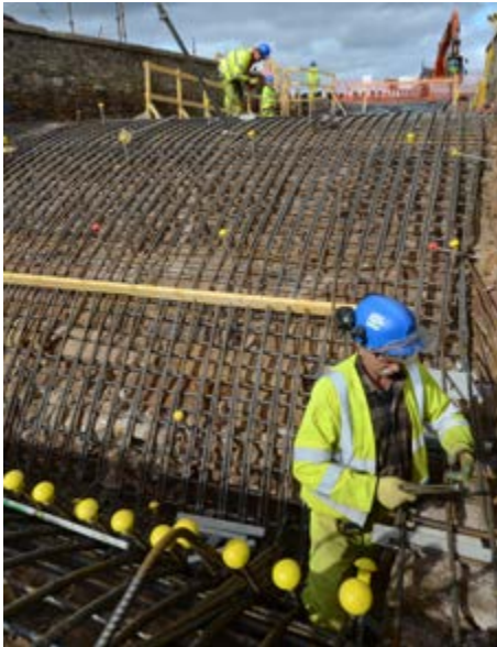
Above Strengthening of the A92 Edenbank Bridge (courtesy of BEAR (Scotland) Ltd)
