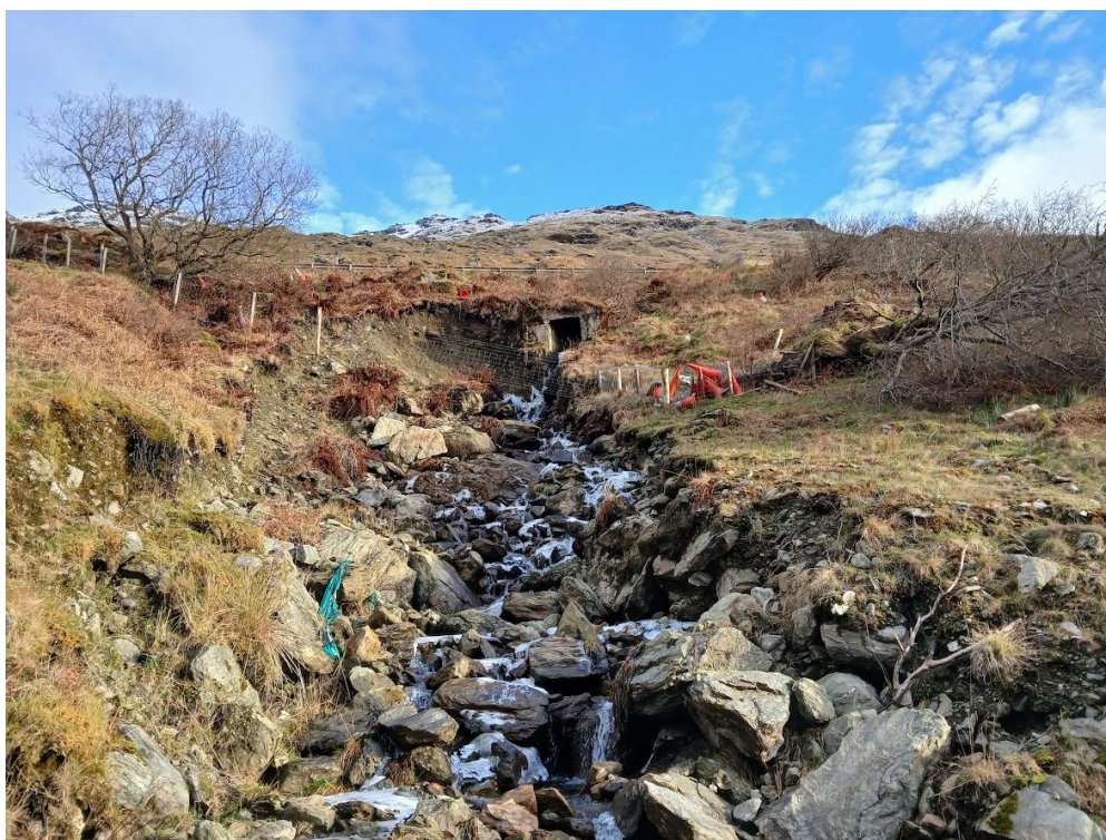
Figure 1: Photo taken in January 2026 showing scour and slope failure downslope of the A83 culvert.
