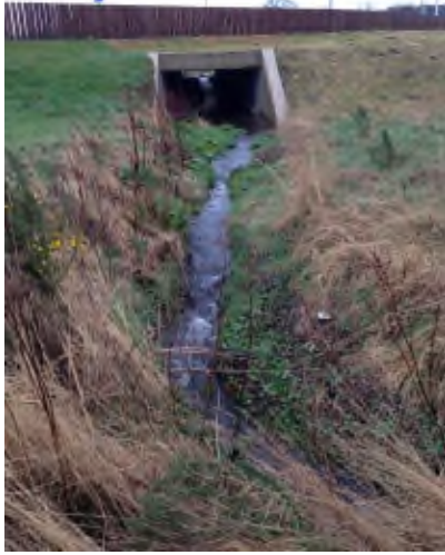
Plate 1: Channel narrowing and laterally adjusting upstream of Highland Main Line
