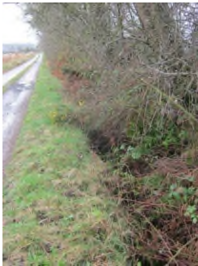
Plate 7: Dry road drain forming part of SWF 07
