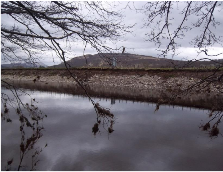
Photograph 11.7: Erosion at ch10000
