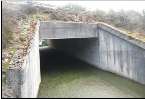
a) West of A9 looking upstream
