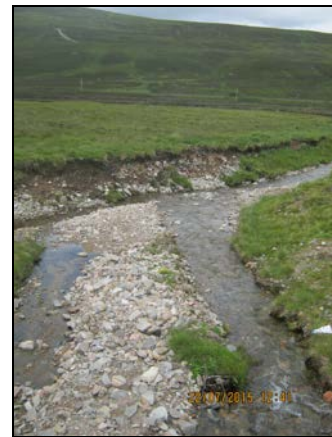
b) Downstream view west of A9, showing bank collapse and a channel bar
