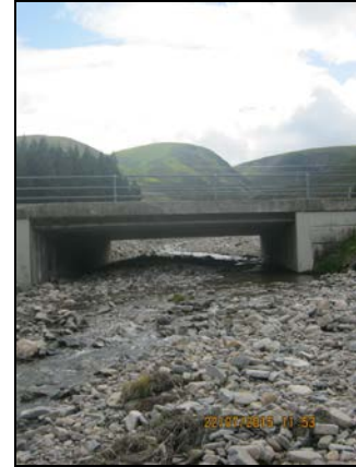
b) Downstream view west of A9, showing pinch-point to sediment movement
