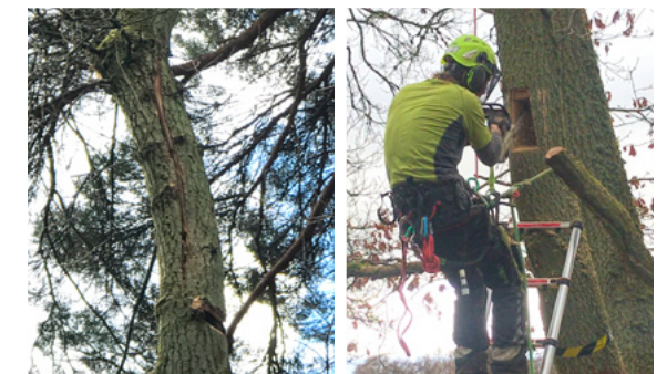
Examples of integrated naturalised tree features (INTFs) and an integrated bat box being created as part of the advance works on Luncarty to Pass of Birnam
