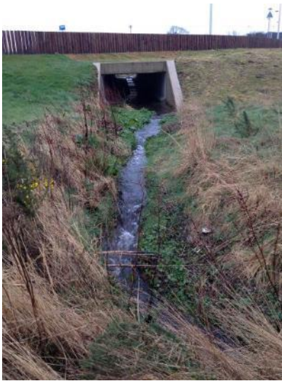
Photograph 3: Straight low flow channel leaving a road culvert at Inverness Campus (NH 69087 44782)
