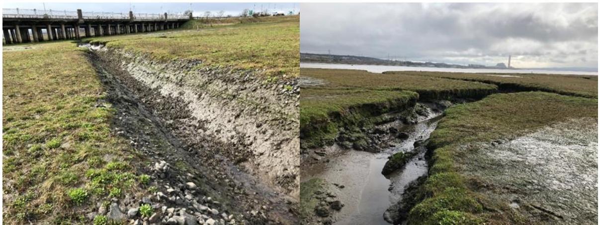
Photograph 1: Existing viaduct and modified creek on northern side of Kincardine Bridge (left) and natural tidal creek south of Kincardine Bridge (right).
