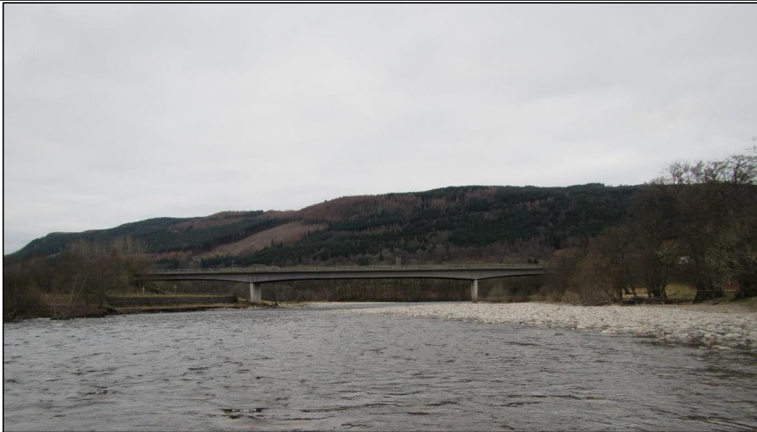
Photograph 1: View of the A9 Tummel Bridge. Photograph taken from upstream of the structure.
