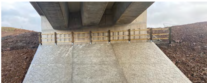
Revetments construction beneath the bridge completing the structure with the installation of kerbs, fencing and staircase.
