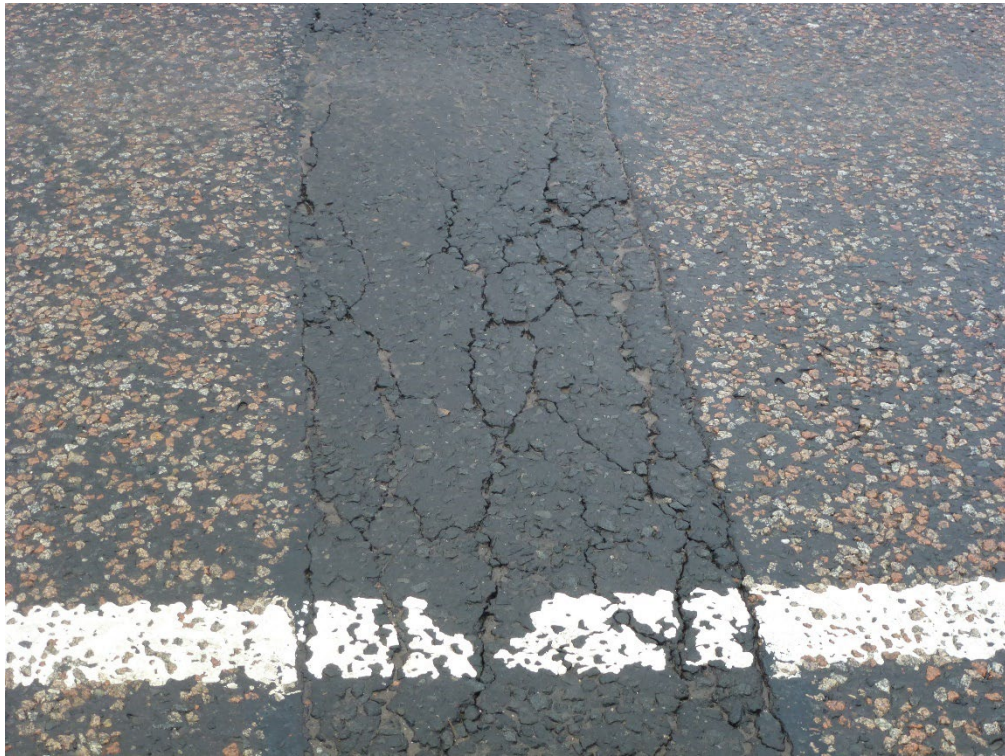
Extensive cracking within reinstatement limits
