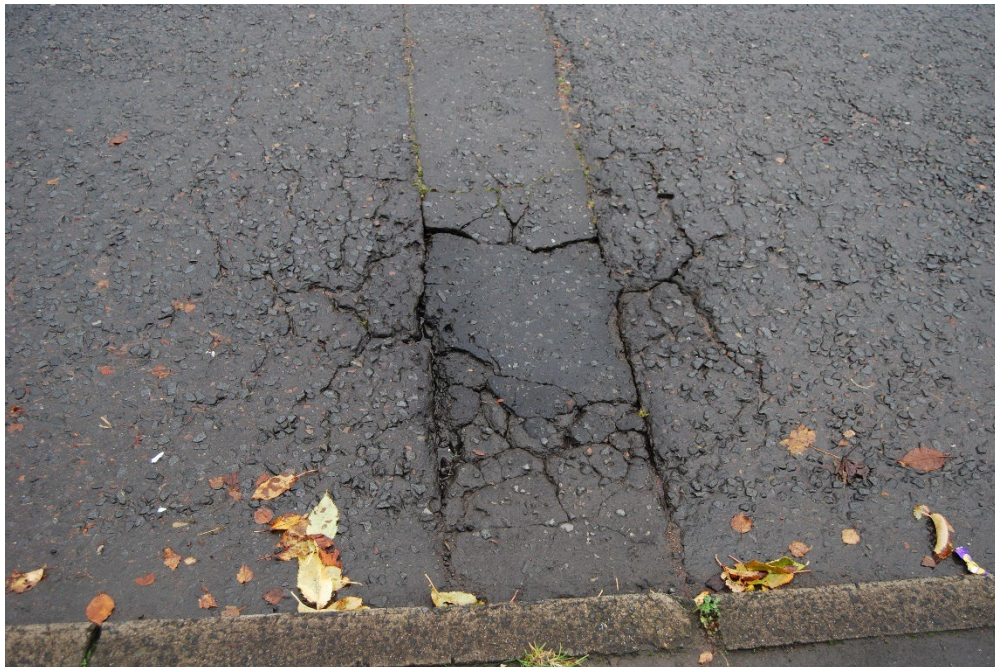
Carriageway cracking caused as a direct result of reinstatement
