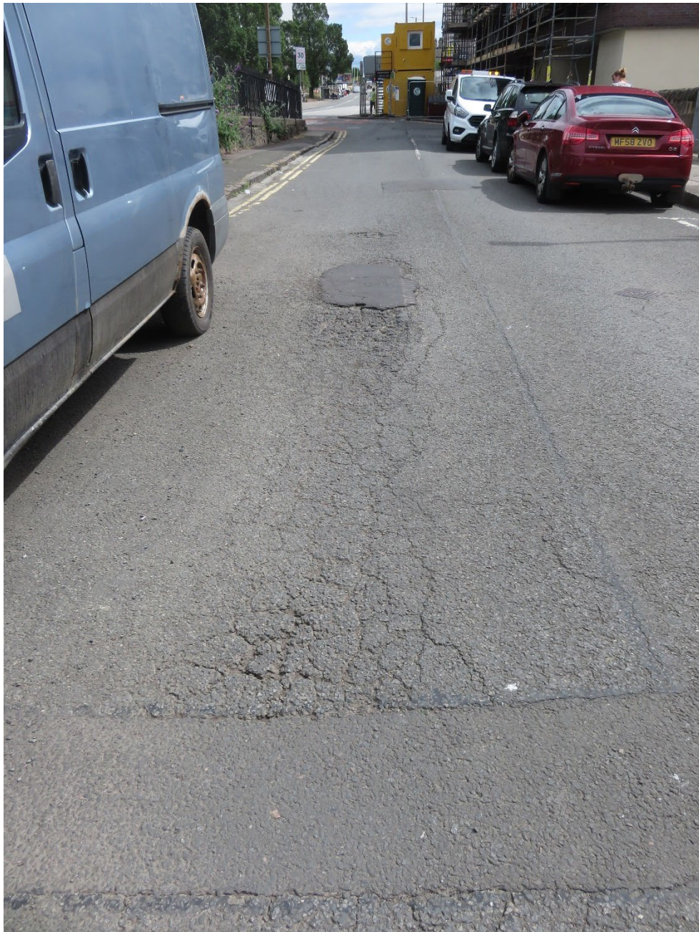
Carriageway cracking that was not caused by reinstatement installation
