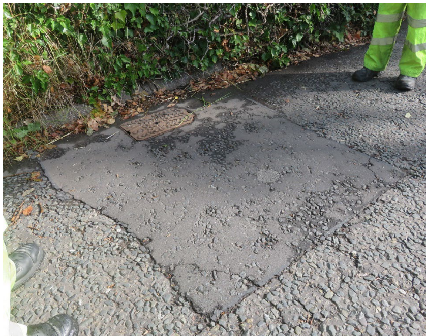
Typical open joint at 4 years
