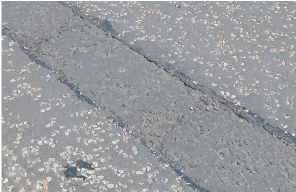
Unacceptable joint – NB associated with aggregate loss, step depression and cracking
