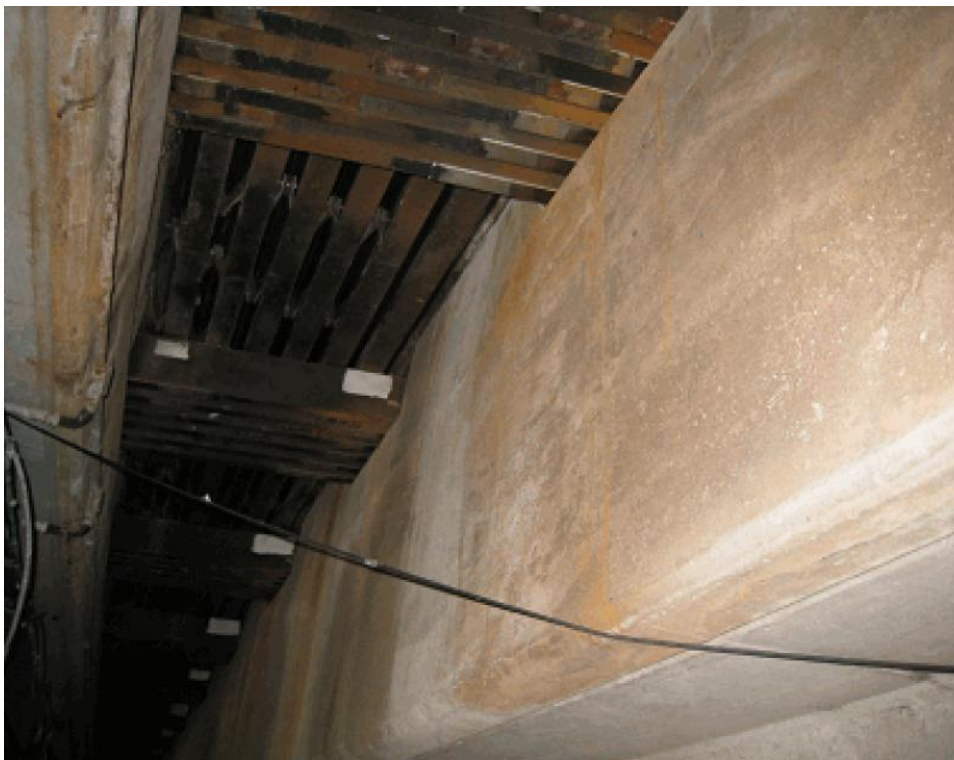
Figure 4 Cable Stayed Bridge (Composite steel-concrete deck) Built 1991 [Rust staining from expansion joints over pier (Seal replacement stopped water ingress.)]
