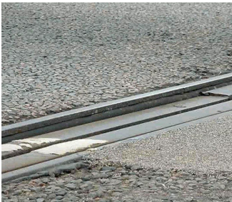
Figure 8 Viaduct (Insitu concrete deck) Built 1986 [ Damage to the West Deck Expansion Joint- Rail broken in the middle and level difference.]
