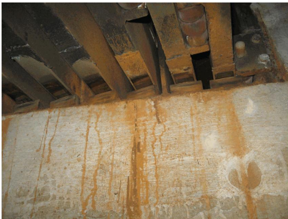
Figure 5 Cable Stayed Bridge (Composite steel-concrete deck) Built 1991 [Corrosion to expansion joints sliding plates over pier.]
