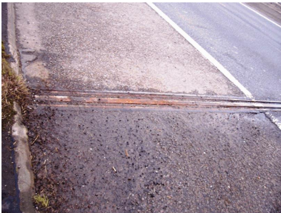
Figure 9 Viaduct (In-situ Prestressed Concrete) Built 1990 [ Corrosion to rails and debris in seals.]
