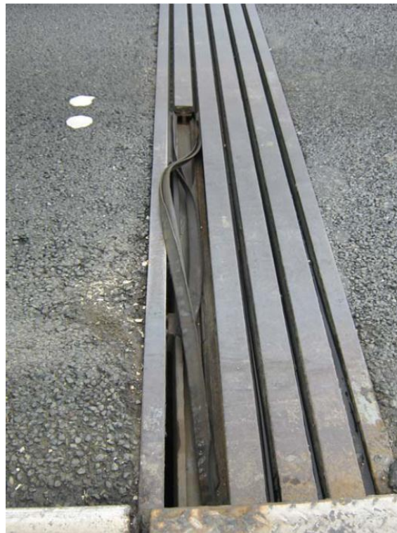
Figure 2 Viaduct (Precast Prestressed Concrete) built in 1993 [The damaged rail has been taken out of the joint and corrosion is visible on the rails.]
