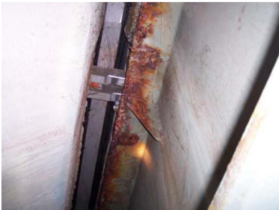
Figure 7 Viaduct (Precast Prestressed Concrete) Built 1976 [ Failure of joint on footway. Seal failed between rails on carriageway.]
