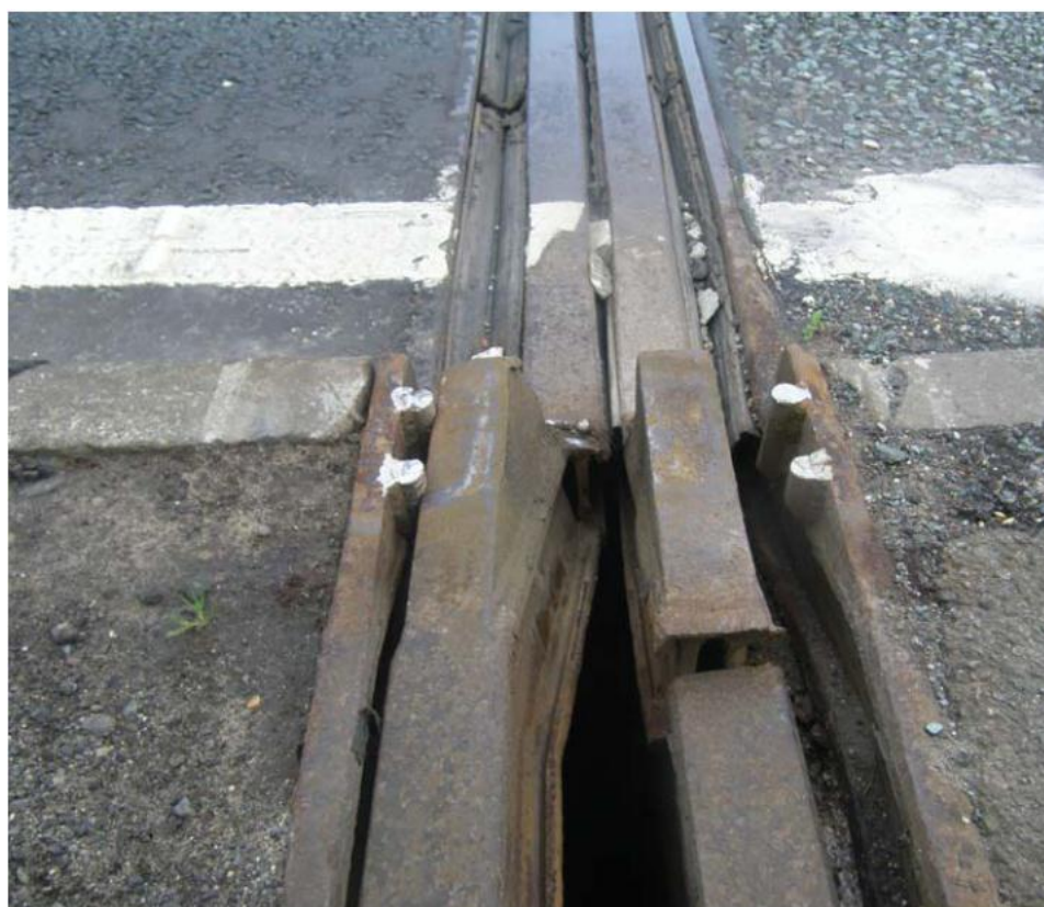
Figure 6 Cable Stayed Bridge (Composite steel-concrete deck) Built 1991 [Trimmer Beam Support Steelwork corroded.]
