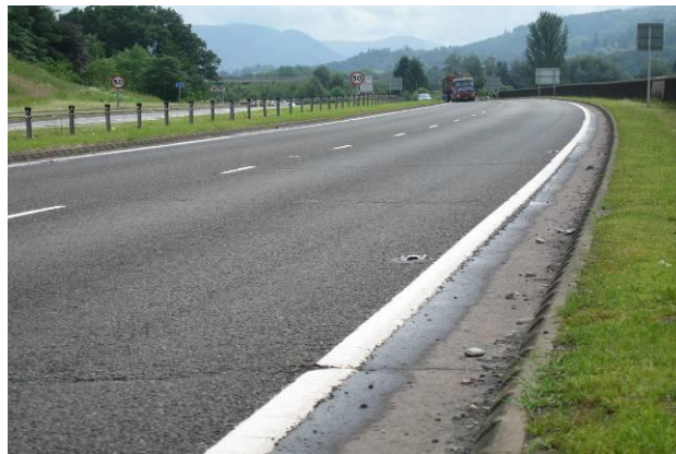
Figure 2.2: Reflection cracking on the A9
