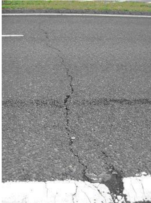
Figure 2.3: Reflection cracking on the A9 near Ballinluig
