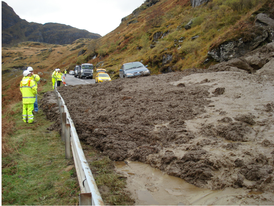
Photograph 1: Disruption to A83 by debris flow
