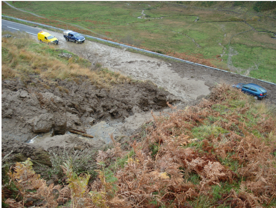
Photograph 2: Looking downhill onto the A83 at the lower section of run-out channel
