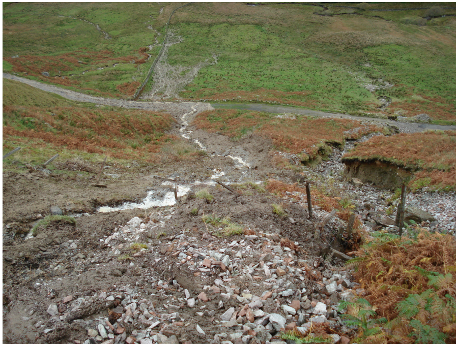
Photograph 4: Debris flow channel below A83. New channel formed by debris flow on left of picture. Previous erosion from culvert on right of picture.
