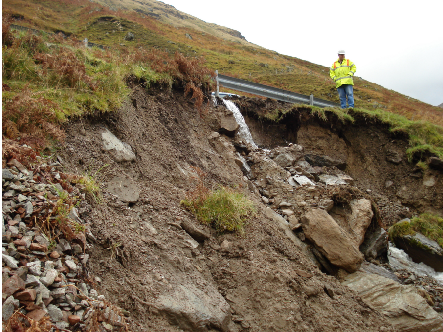
Photograph 3: Undercutting of A83 by debris flow and surface water erosion
