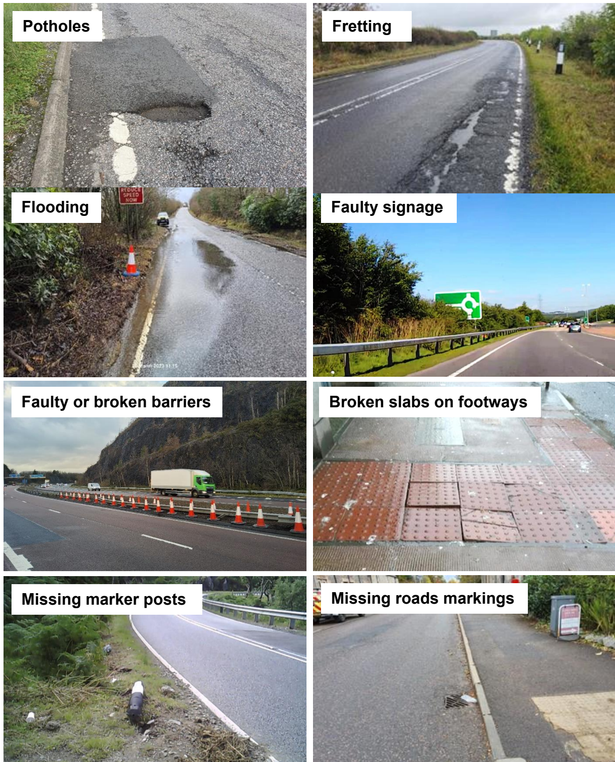
Figure 2.12: Images of defects shown to respondents
