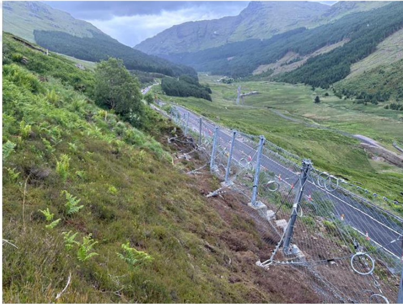
A83 RABT Landslide Barrier
