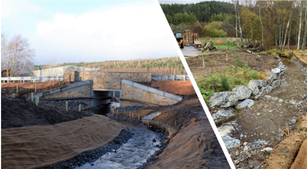
Figure 48 Upstream view (left) and rock armour and coir rolls installed around the new structure (right) on the A887
