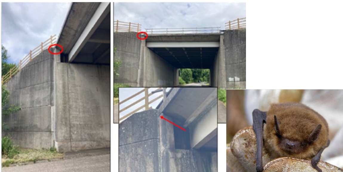
Figure 33 Bat roost locations (NW corner of the bridge) and a common Pipistrelle bat (image from Amey)
