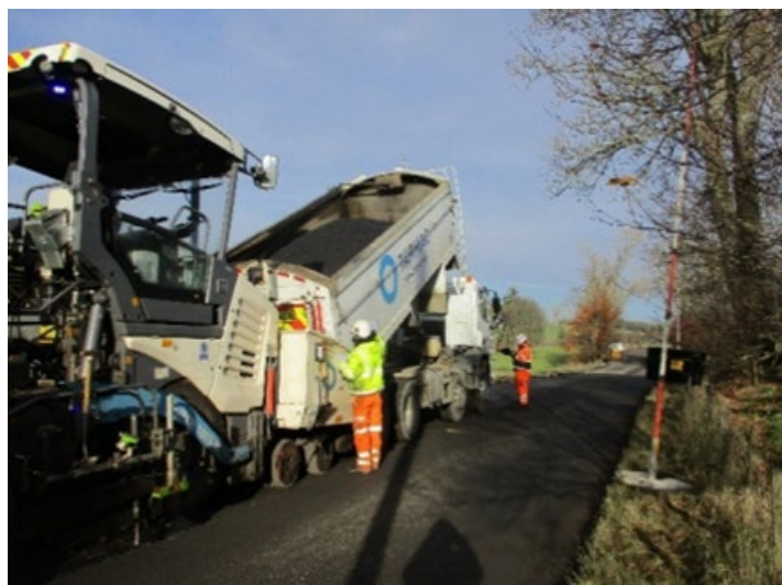
Figure 52 A702 Lamington where the existing road tar has been stripped, processed and re-laid
