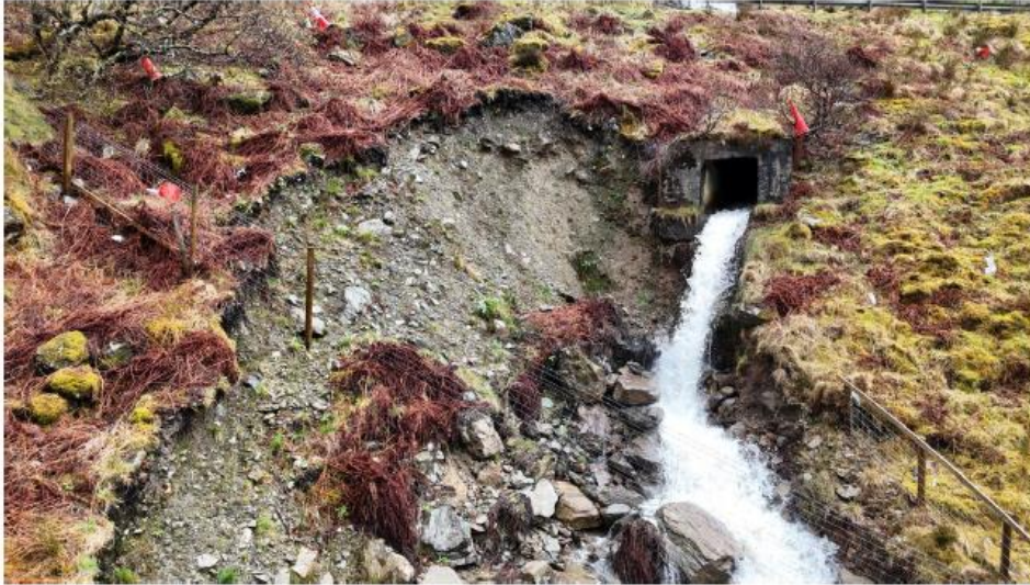
Lower Slope Scour
