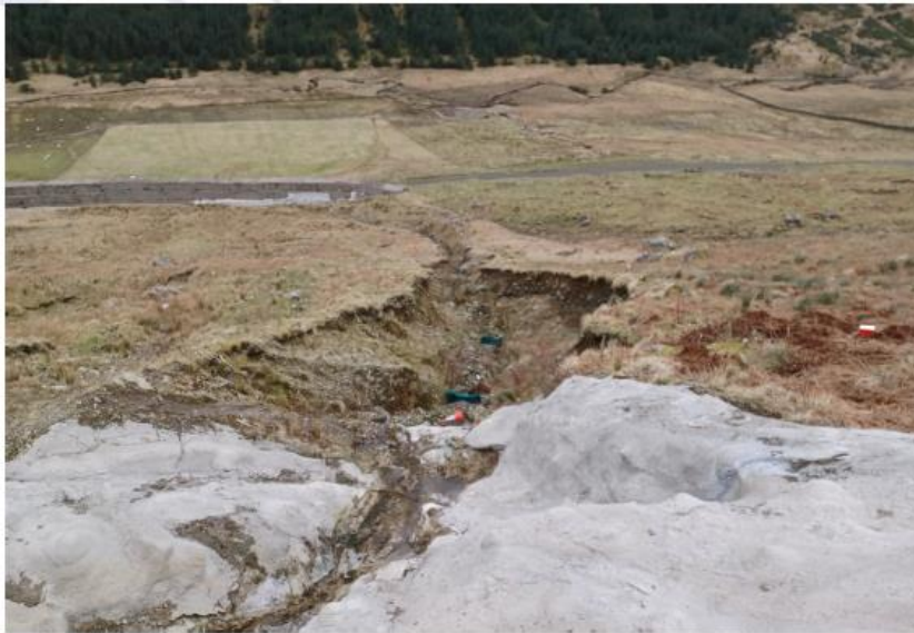
Lower Slope Scour
