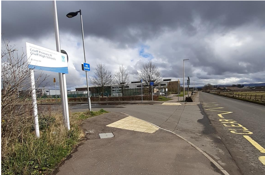
Figure 10: New drop kerbs and tactiles installed on Broich Road near the main entrance to the Crieff Primary and High Schools in Crieff (Image © Perth & Kinross Council)
