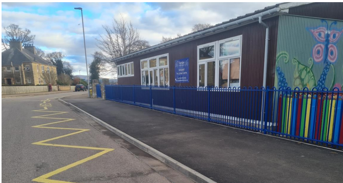
Figure 13: A relevant example of minor measure delivery of a full footway resurfacing in front of Bishopmill Primary in Elgin, not the direct result of a school route audit (Image © Moray Council)
