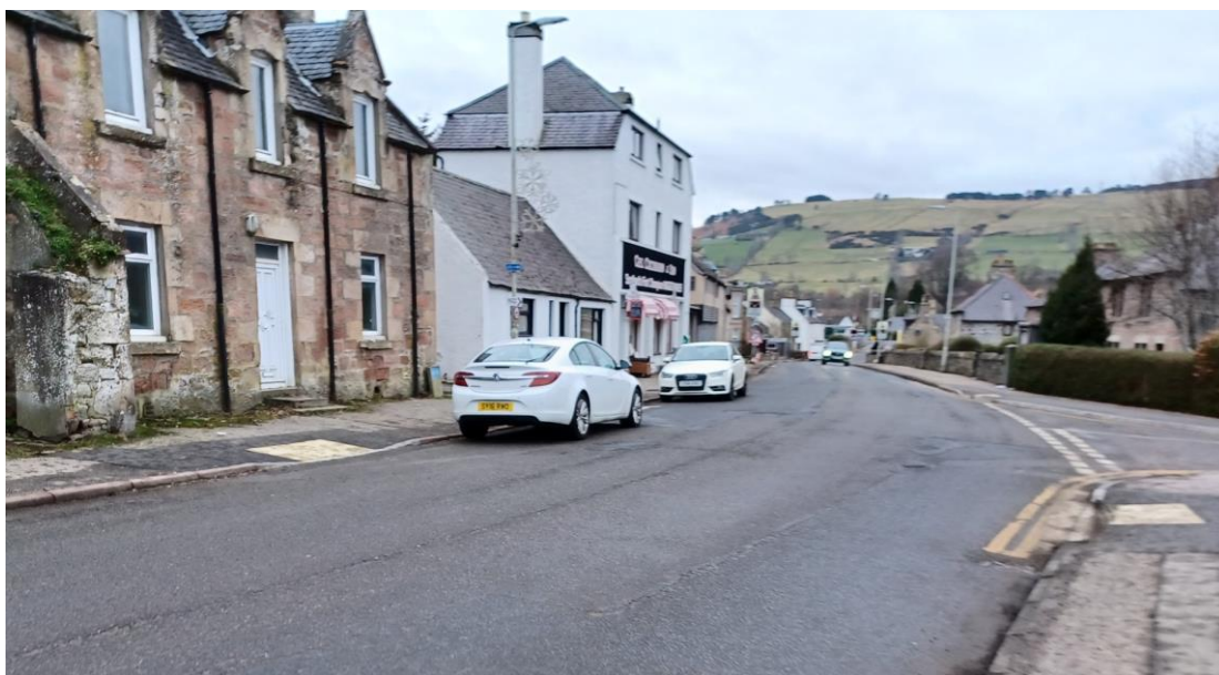
Figure 7: New drop kerbs and tactiles installed on Mill Street, Dingwall © Highland Council
