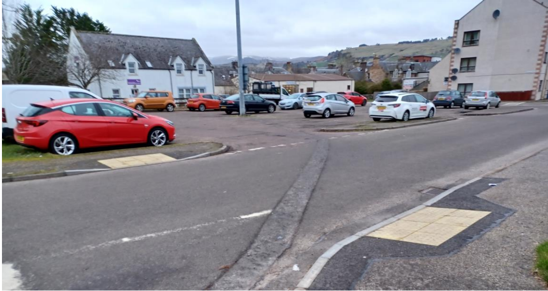
Figure 8: New drop kerbs and tactiles installed off Hill Street in Dingwall (Image © Highland Council)
